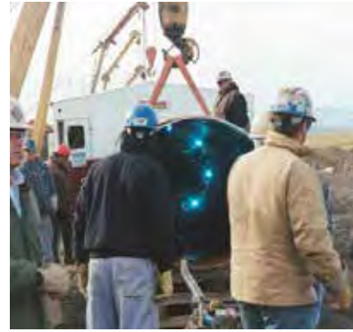
Figure 14. Gas Metal Arc Welding (Westpath, internal welding of the Gr. 690 using the 4 head, short circuit GMAW [7].)
